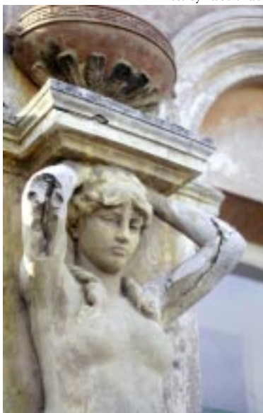
Exposed iron structure on the caryatid.
